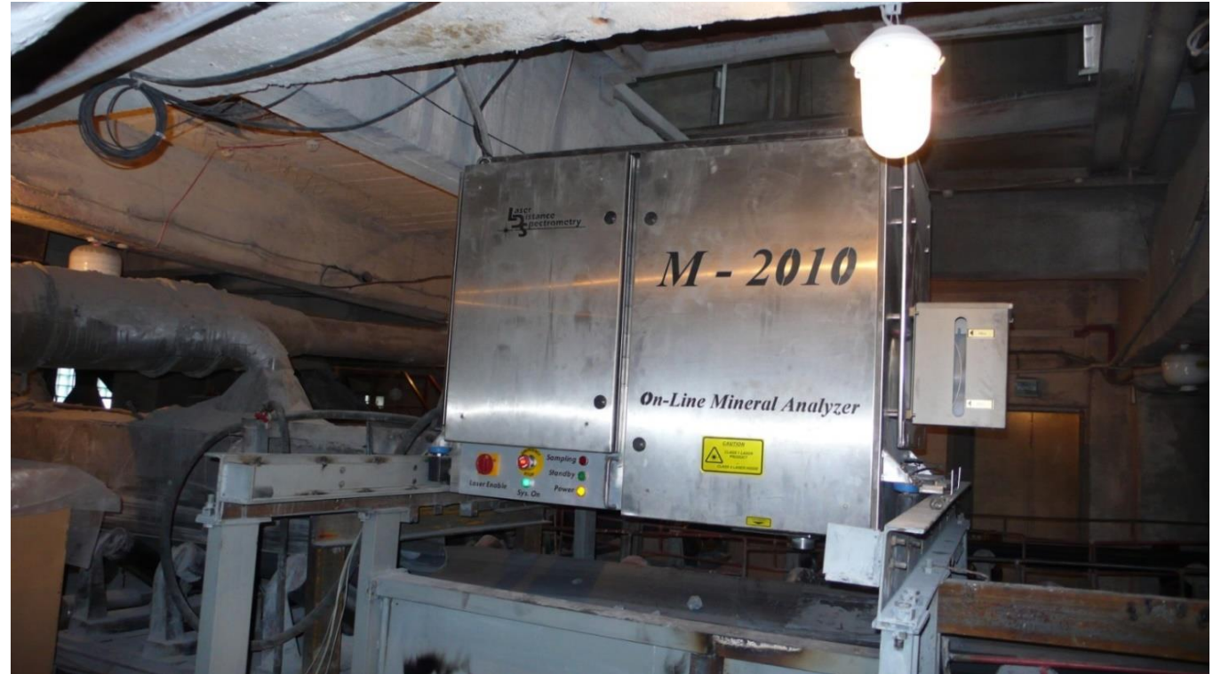
Ore Online Elemental Analyzer above a conveyor
